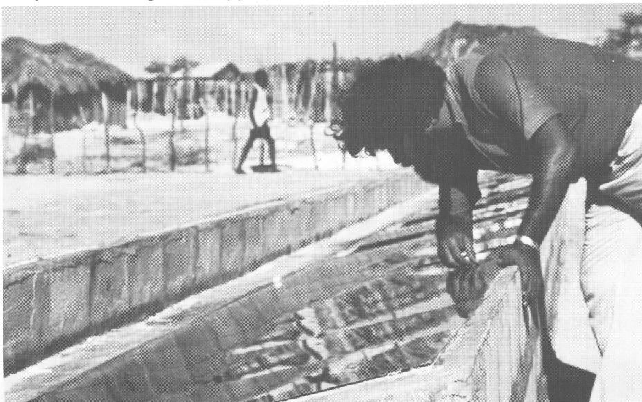
Frank Malvar of TAL works on construction of 35-square-meter solar water still at Tit Anse, Haiti. The huts in the background are typical village housing.
