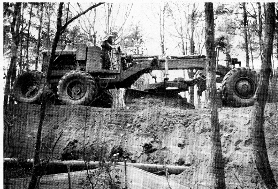
An Air Force Heavy Equipment School student works on the sediment pond dam at the Cobb County far-field antenna range site. An exposed section of the six-inch conduit for the data link can be seen at the bottom of the photo.
