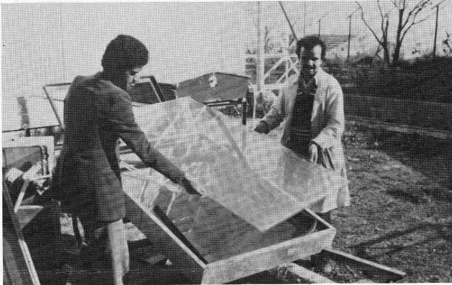
Algerian researchers construct a modified passive solar air heater at the Station de l'Energie Solaire near Algiers. The North African country is starting a crash program to develop solar energy and one of their consultants in the effort is Georgia Tech scientist J.D. Walton, Jr.
